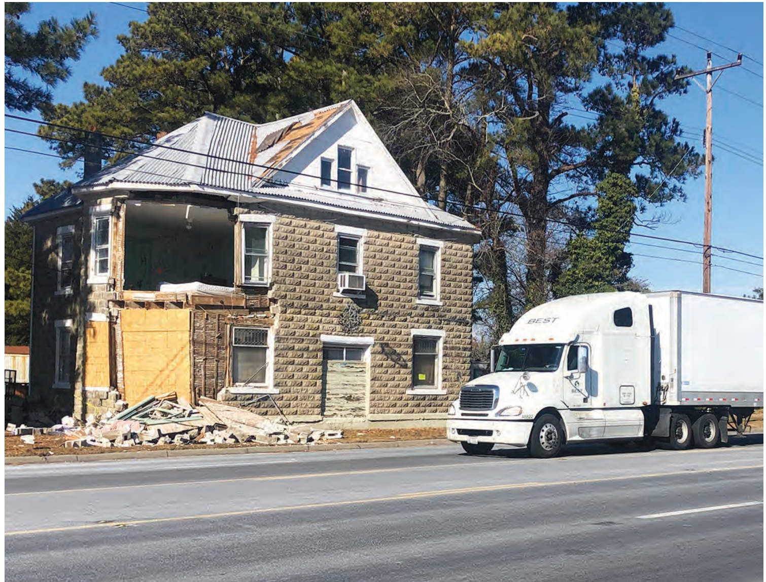
EASTERN SHORE POST/TED SHOCKLEY A southbound truck passes the Adney residence at 33372 Lankford Highway, Painter, which was hit by a vehicle on Oct. 21, 2024. Pieces of the home have fallen into the highway since the crash, prompting officials to close a lane of traffic.
