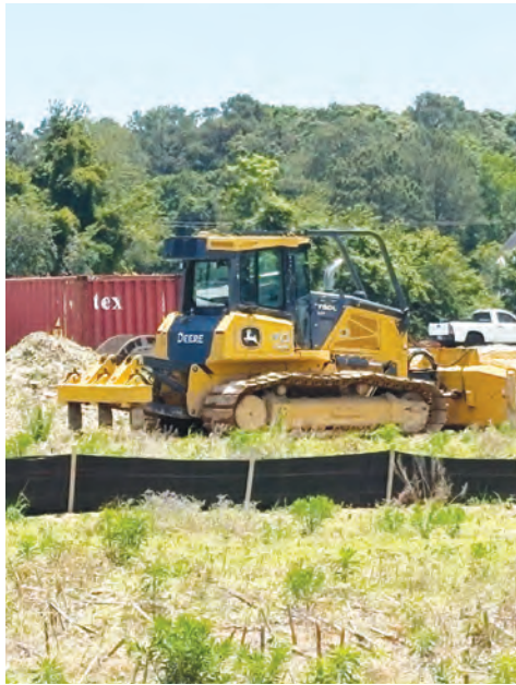
EASTERN SHORE POST/TED SHOCKLEY Equipment sits on property near Wattsville where Accomack County ended construction on a electricity storage facility.
